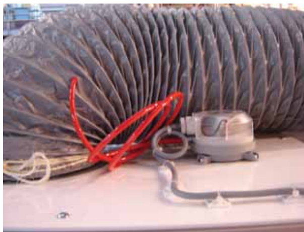
Figure 3.11: Safety module in the exhaust tube of the plasma unit
